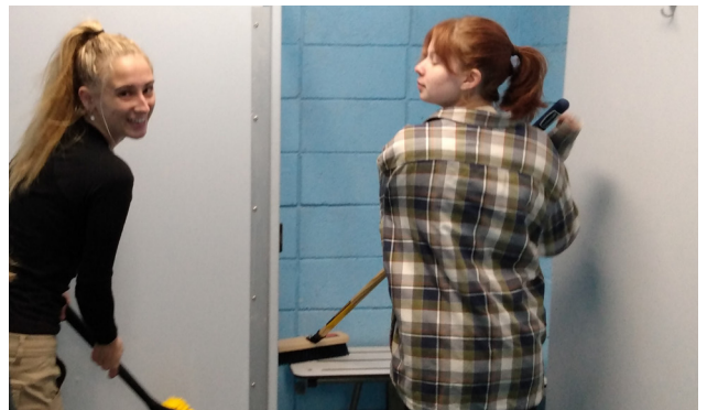
Prepping bathrooms for painting for the renovation at the Allen Rosen Aquatic Center.
