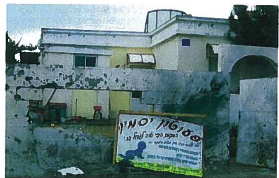
A building recently damaged by a missile in Sderot.
