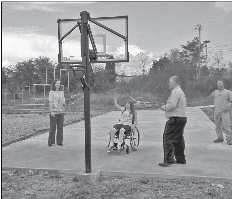
Sarah Perez taking the first shot at the new basketball hoop! Our new playground is under construction!
