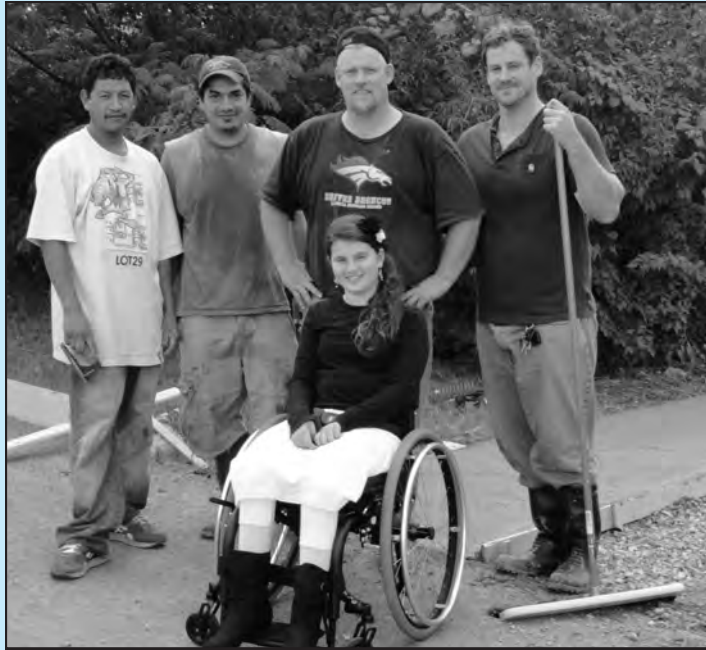
John Cass, his son Billy, and two of his crew, pose with Sarah by the new sidewalk they installed for KJDS.
