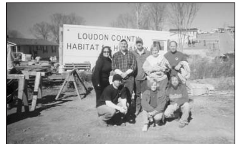
A hardy crew prepares to work on a house at the Loudon County Habitat for Humanity project.
